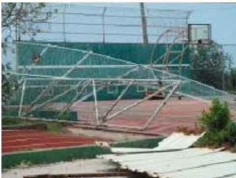
Collapsed fencing on a basketball court
