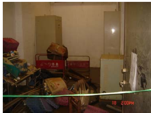
A flooded switching room
