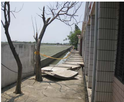
A collapsed wall
