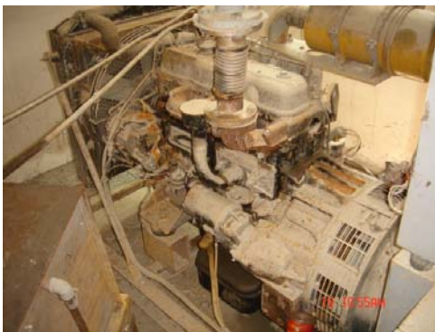
A flooded generator
