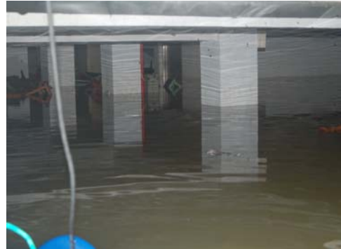
Flooding in the basement level
