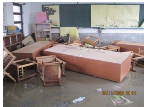
A flooded classroom
